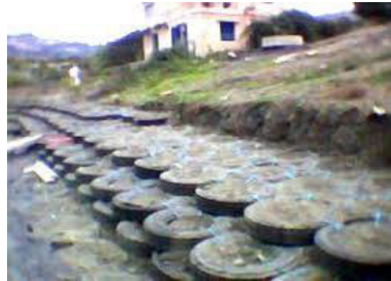
Figure.1.2. Stability of a landslide - Tizi ousou.
