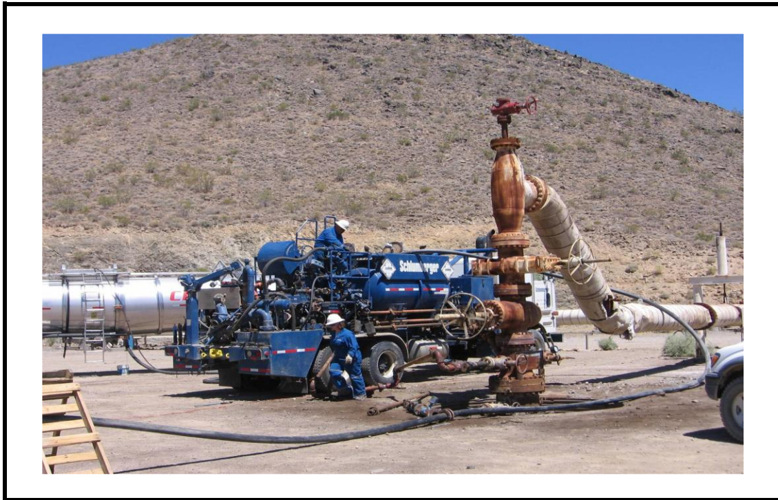
Figure I- 1: Installation of a pumping unit for injection of chemical compounds [18]
